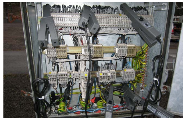
Figure 3 Control cabinet with current clamps
